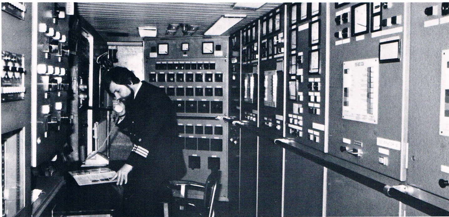
Maschinenzentrale • Engine control station
