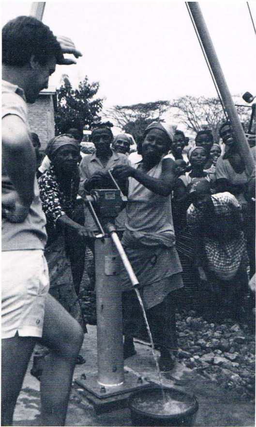
Ghana, Herbst 1981, von GEOMECHANIK gebohrter Brunnen mit Handpumpe Ghana, autumn 1981, a well with hand pump, drilled and installed by GEOMECHANIK
